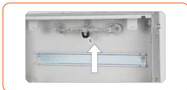
Remove link to use split neutral provision • Use 1st neutral link for mains supply • Use 2nd neutral link for stand by supply
